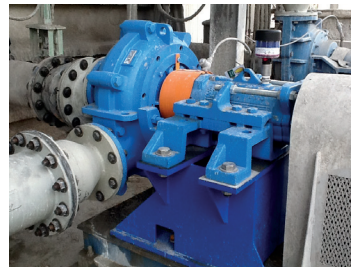
Ball mill discharge in Phosphate plant
