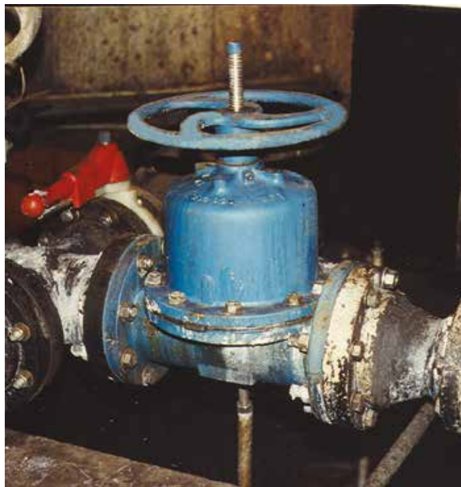
Straightway Valve on Abrasive Slurry Service
