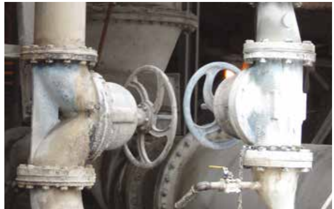
Weir Type Valve in Phosphoric Acid Service
